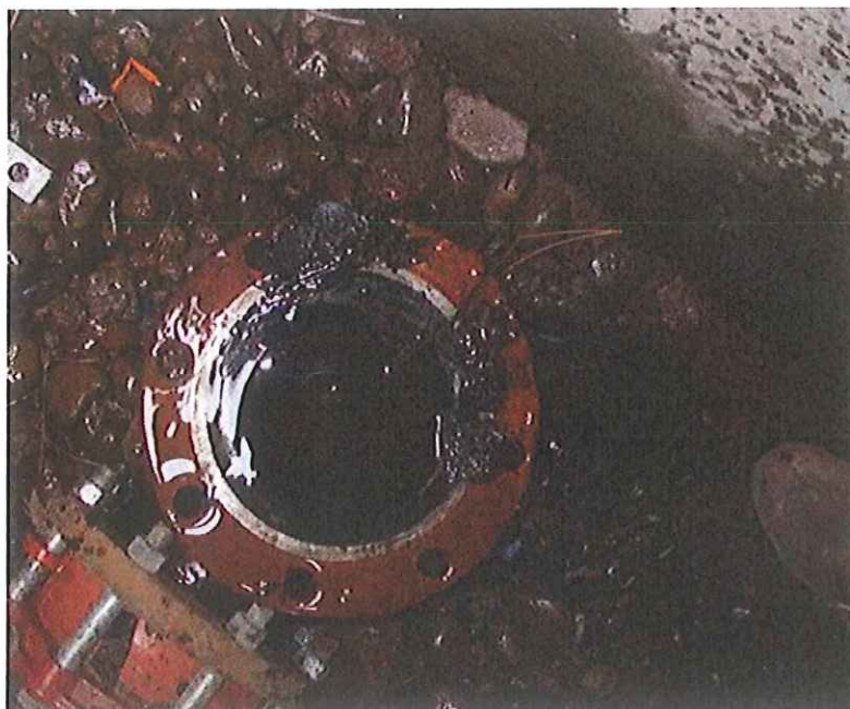
Figure 1. An accumulation of pipe lining material (black material) with sand and gravel in one of the Outback reservoirs
