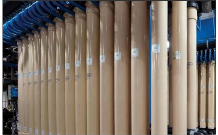
Typical water membrane filtration racks, similar to what is being constructed at the Water Treatment
