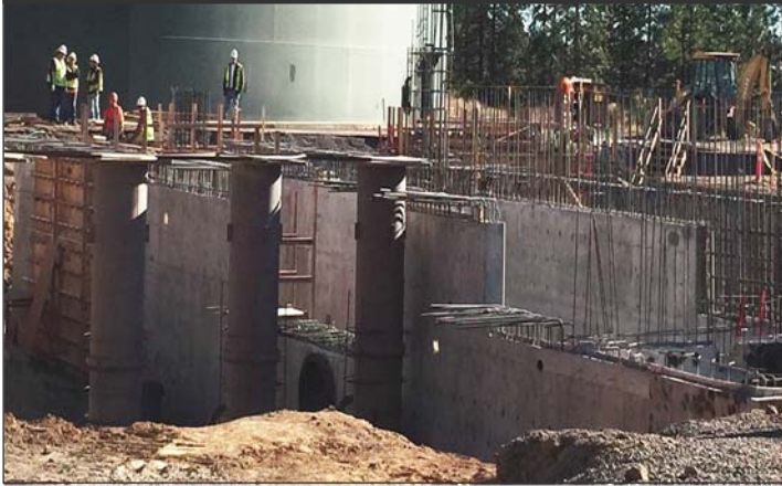
A current picture of the water treatment plant foundation, pipe gallery and underlying infrastructure
