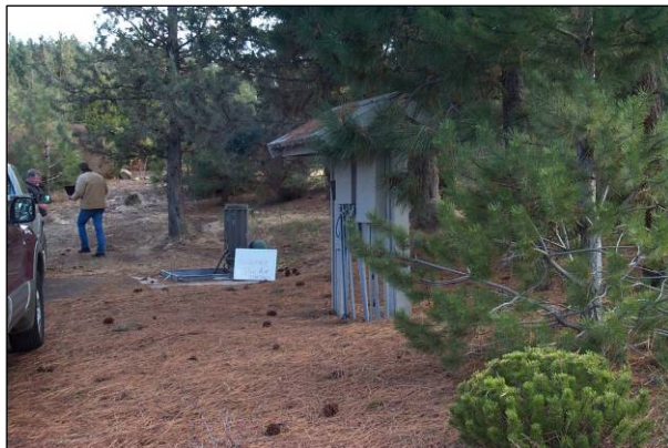
Figure 12: Awbrey Glen PS Air Station
