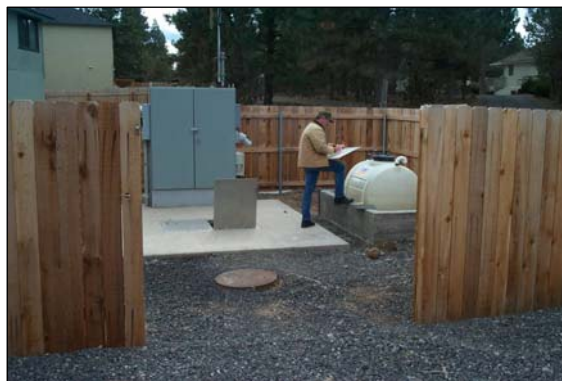
Figure 24: Deschutes County Jail Pump Station
