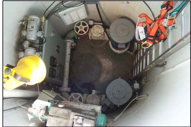
Figure 29: Inside Drake Pump Station Dry Well
