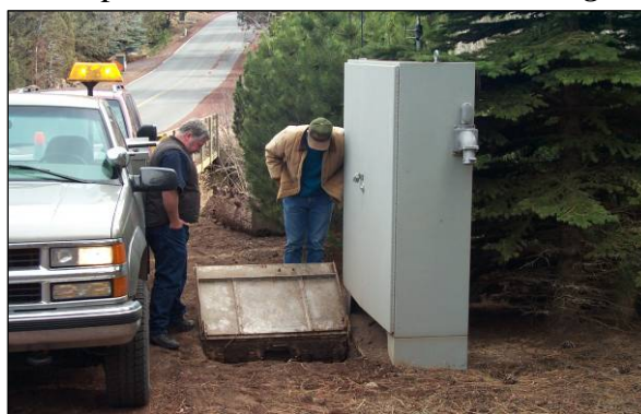
Figure 16: Wyndemere Pump Station
