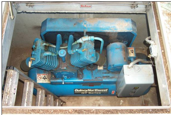
Figure 13: Awbrey Glen PS Air Station Compressor
