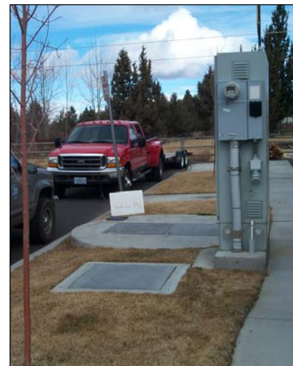
Figure 20: Boyd Acres Pump Station
