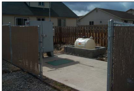
Figure 25: Majestic Pump Station
