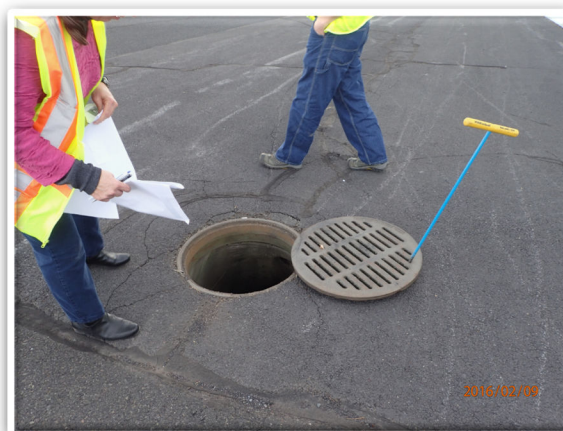
Conducting open grate drywell inspections as part of the UIC Retrofit Project.
