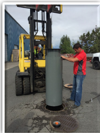
Installing open grate UIC retrofit at Boyd Acres corporation yard as an installation demonstration.
