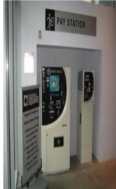
Example: Pay on Foot in elevator lobby – Fountain Square Garage, Cincinnati OH
