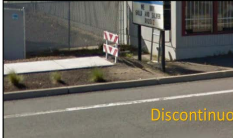
Non-Compliant Curb Ramps
