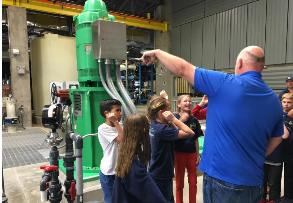
Rod Mingus explains feed pumps at the Water Filtration Facility to St. Francis students.
