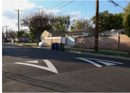
Example of speed hump
