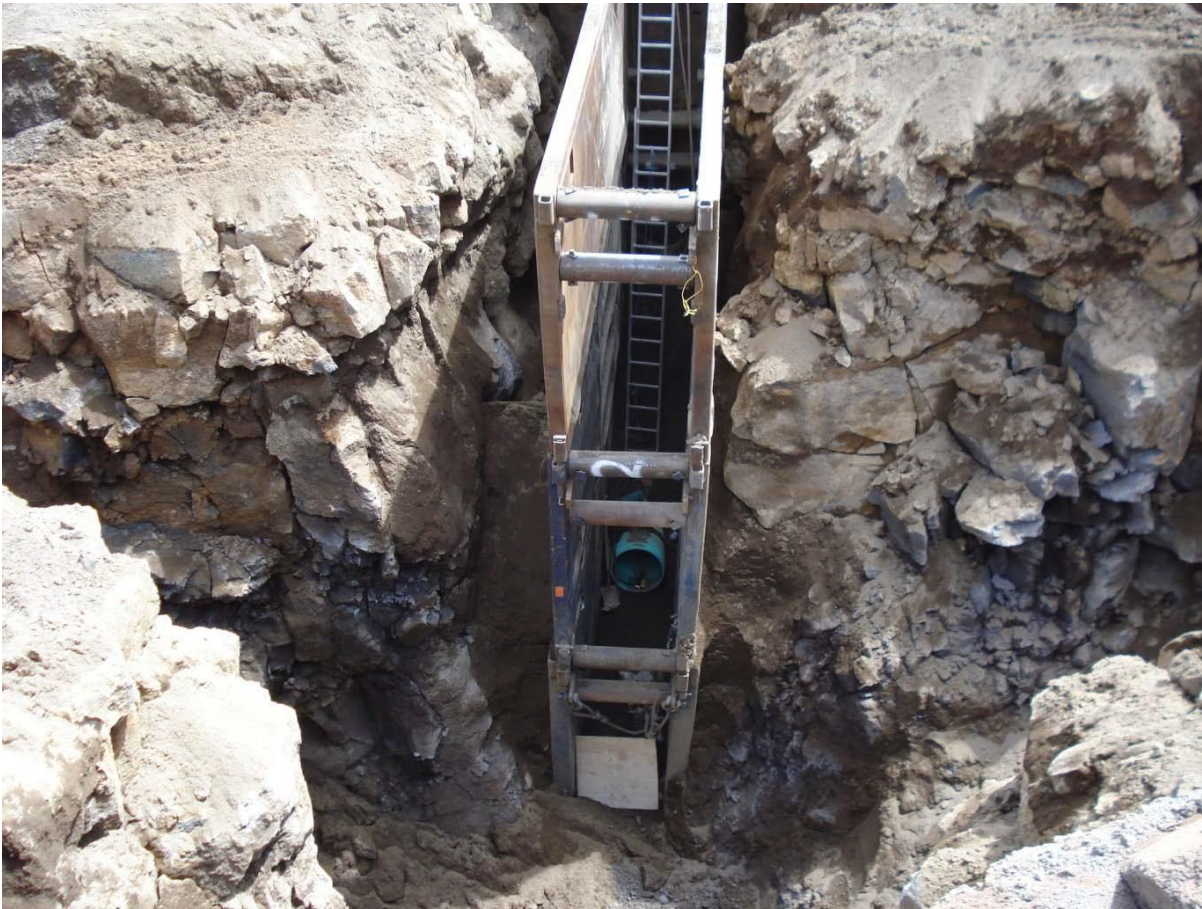
FIGURE 5 Murphy Road Trench Support (24-inch gravity sewer approximately 25 feet below existing grade – presplitting and controlled blasting employed)
