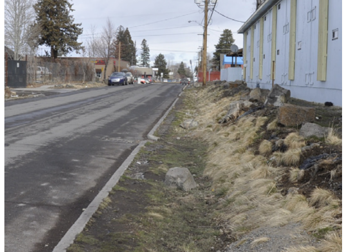
Missing sidewalks in residential and industrial areas
