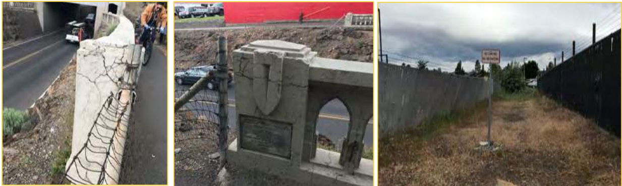
Crumbling concrete at the Franklin Street underpass and chain link fences with barbed wire are some of the aspects of the area survey respondents would like to see improved.
