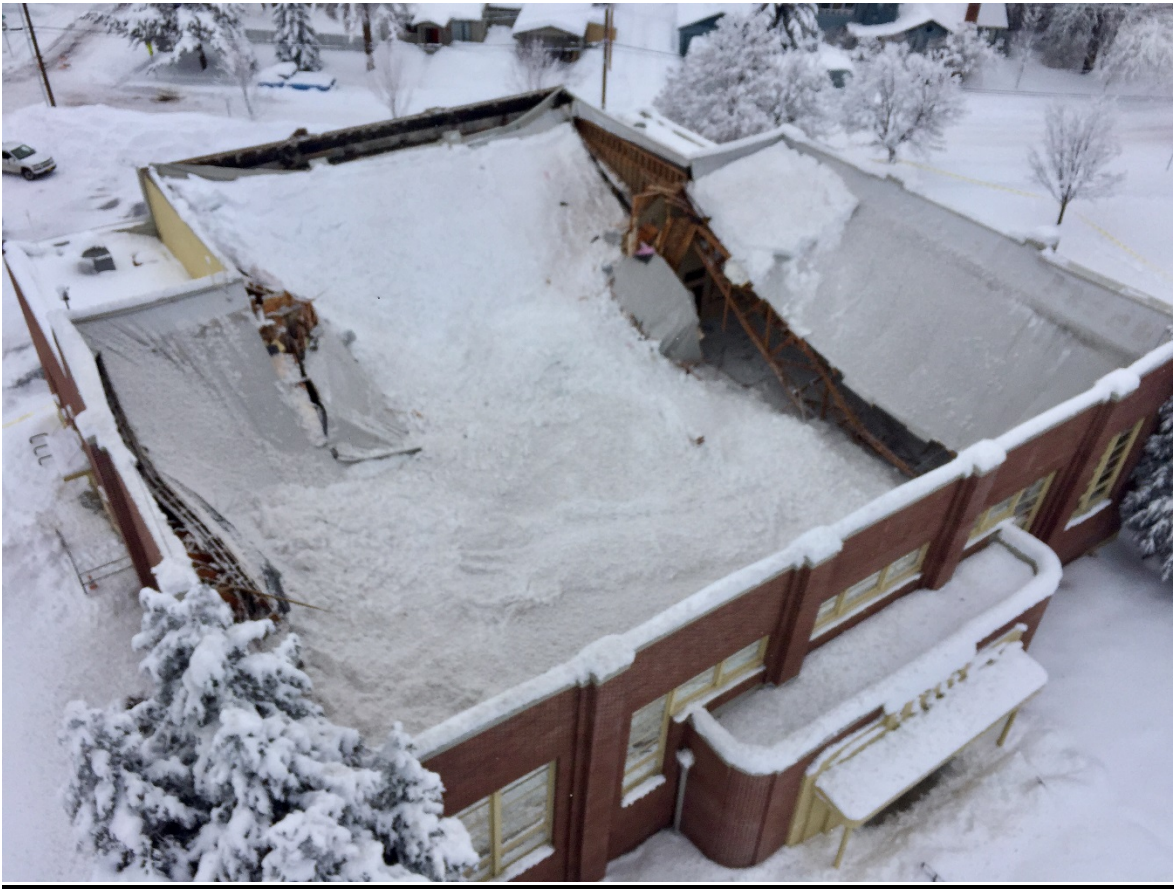
Highland School (Kenwood) gym roof collapse, 2017
