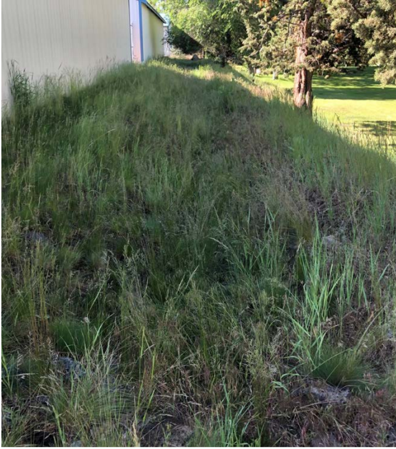
Swale vegetation needs cut and pipe outlet cleared.
