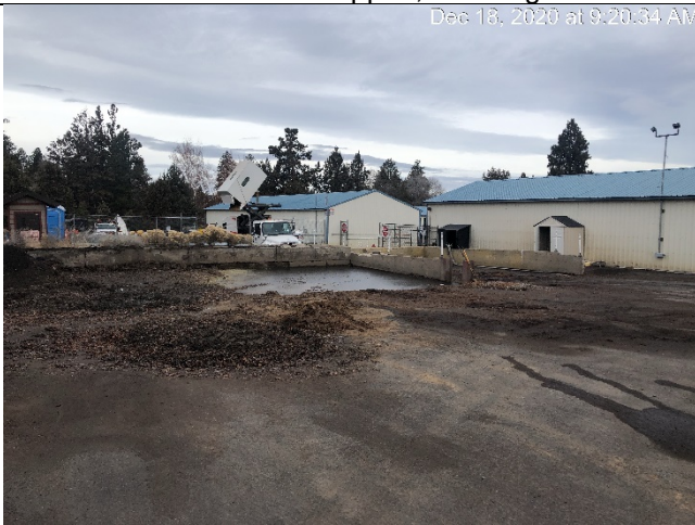
Sweeper decant area drain not draining.
