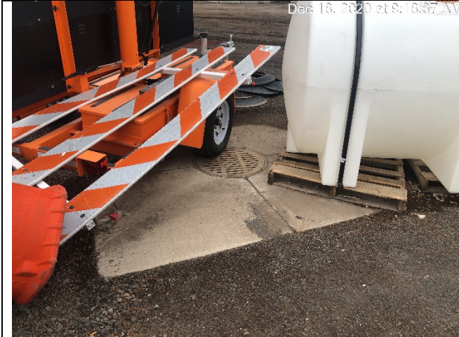
New catch basin needs mapped, discharge location is unknown.
