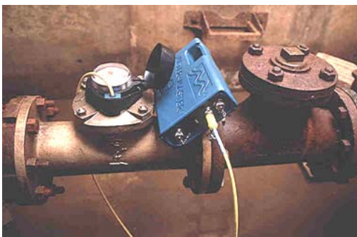
Meter-Master flow recorder installed on a magnetic drive water meter. (Photo courtesy of the F. S. Brainard Company)
