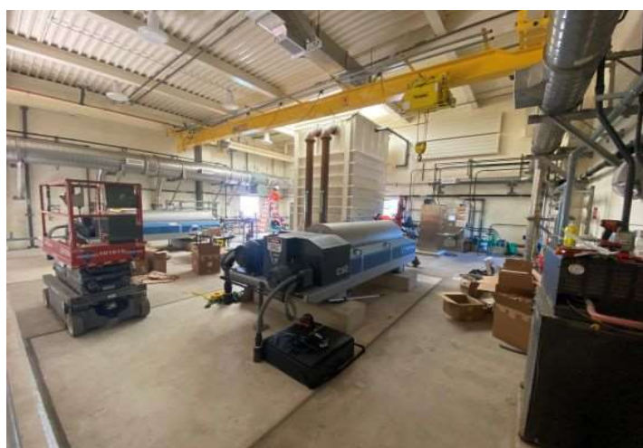
This photo shows the two new centrifuges along with the new bridge crane on the mezzanine floor of the solids building. Photo taken fall of 2021
