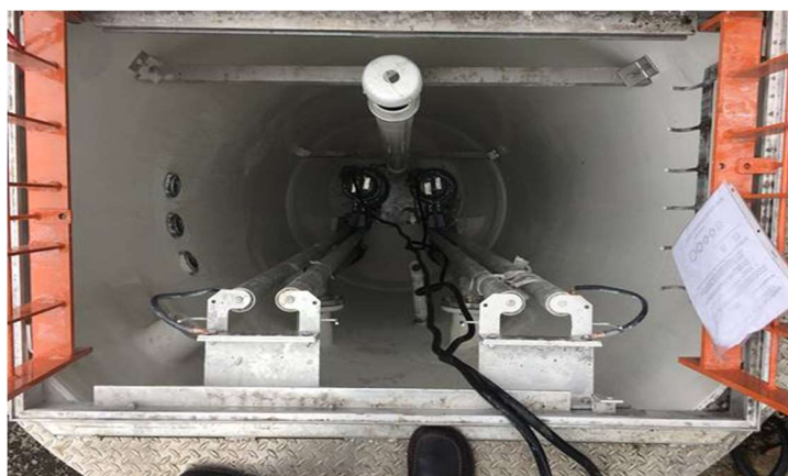
Pump station wet well
