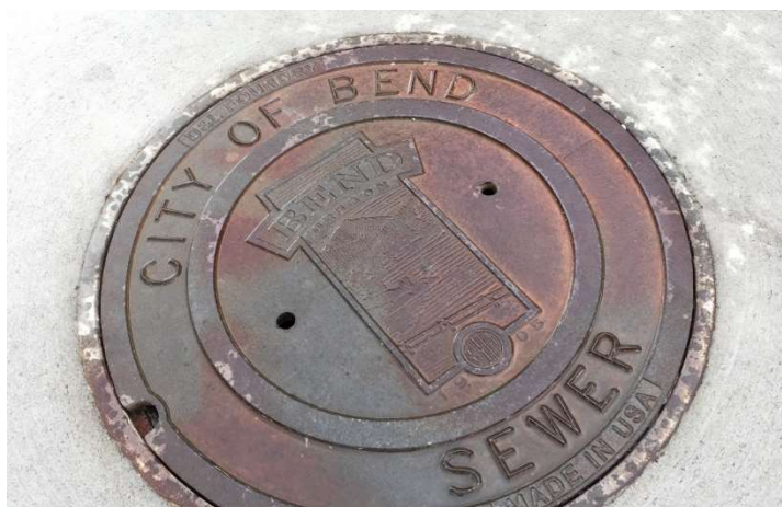
City of Bend standard collection system manhole lid.
