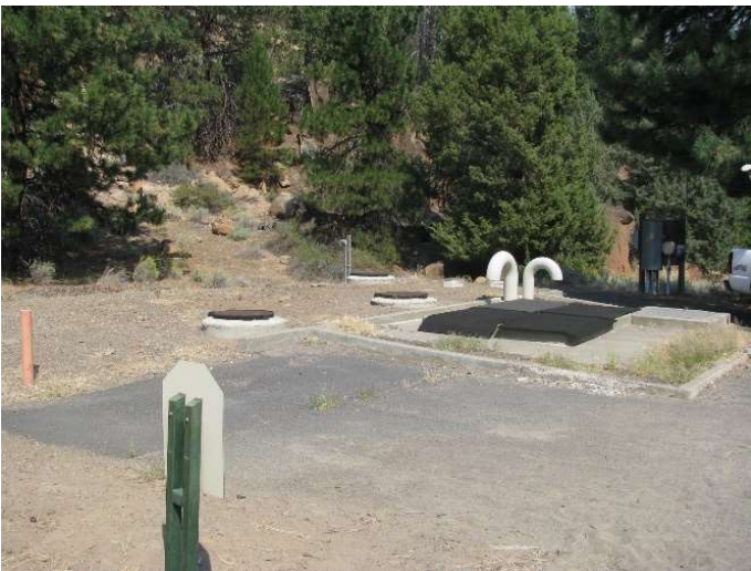
Awbrey Glen Pump Station
