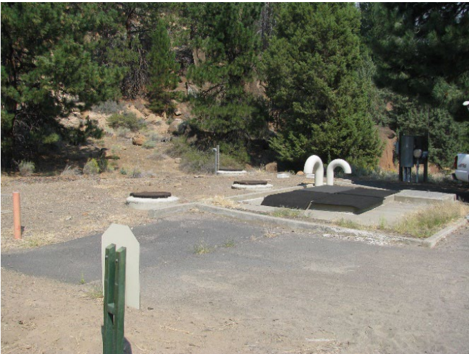
Awbrey Glen Pump Station
