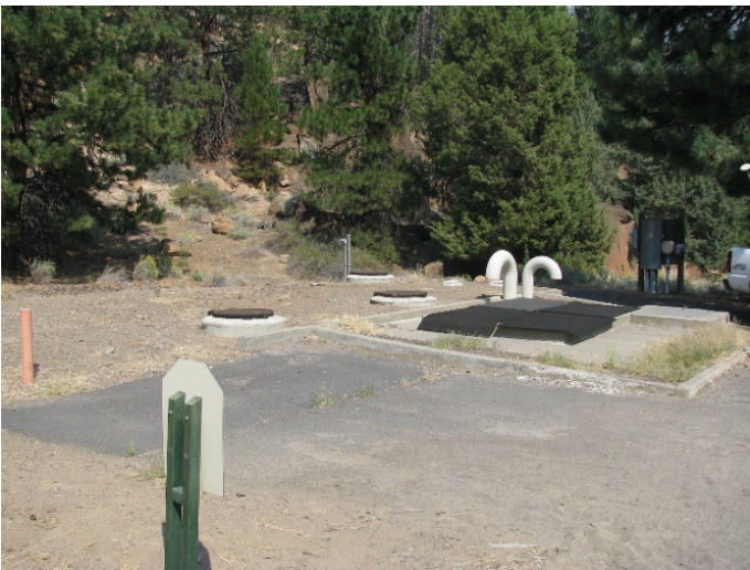
Awbrey Glen Pump Station
