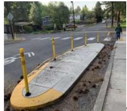
Figure 9. Vertical delineators used to inform drivers and plow operators of obstacles, and gap in curb extension design that requires additional maintenance.
