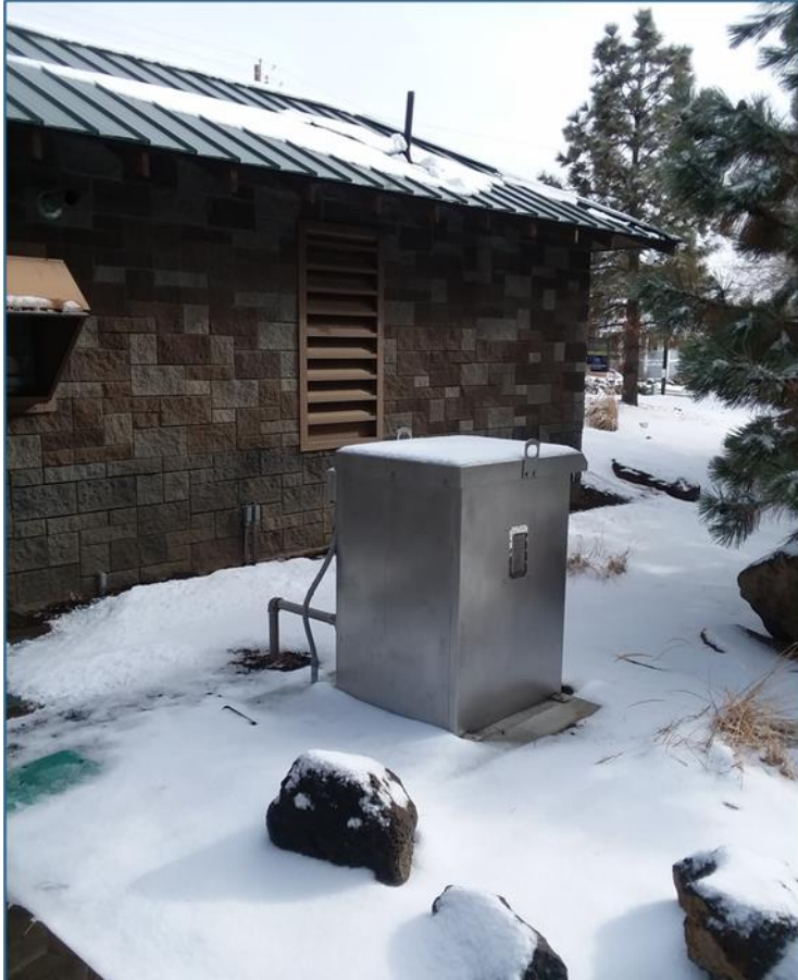
Sawyer Park Pump Station
