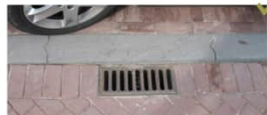
Detail of a good application of a 45x20 street gully with roller layer
