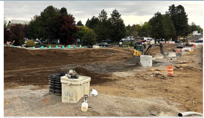
Newly installed utility vault and manholes for stormwater and sewer are set at the final roadway height along Neff Road.
