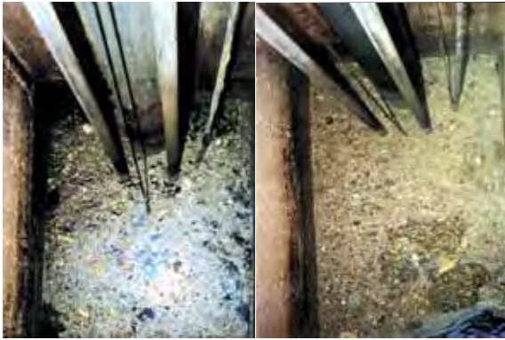
1-Typical influent of pump station with floating scum. Pump "Off"
