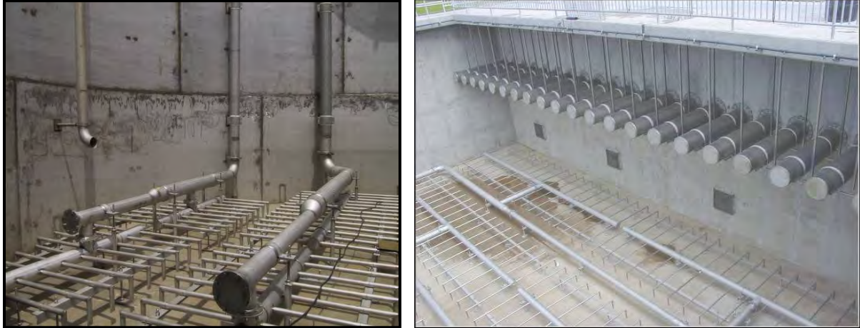
Figure 1. Diffuser grid assemblies in a moving-bed reactor.
