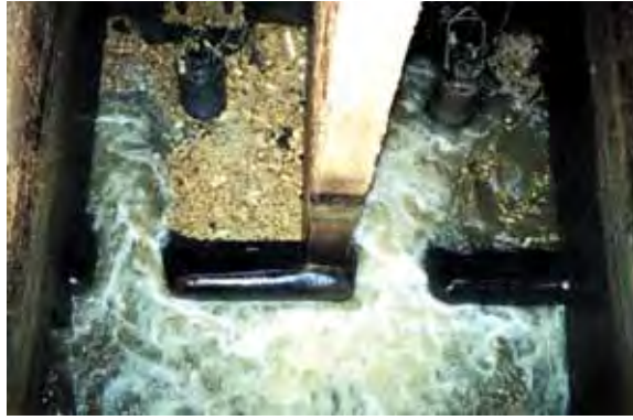
4- Floating material is entrained and folded into pump suction by prerotation action and pumped from wet well.
