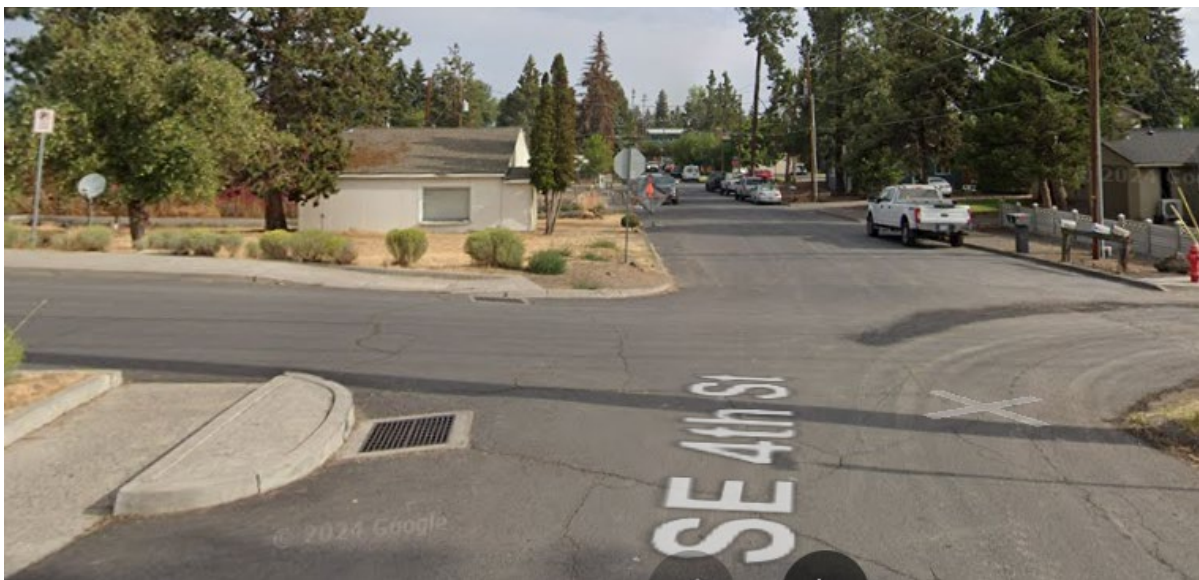
4 th Street Missing Sidewalk
