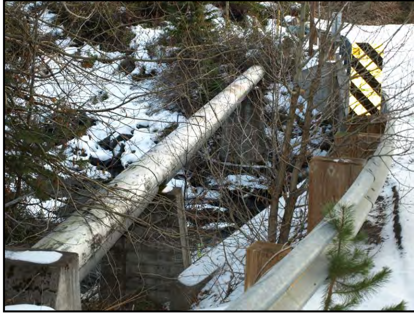
Figure 7.25. The 1957 pipeline crossing Tumalo Creek immediately adjacent to the Forest Service concrete bridge.
