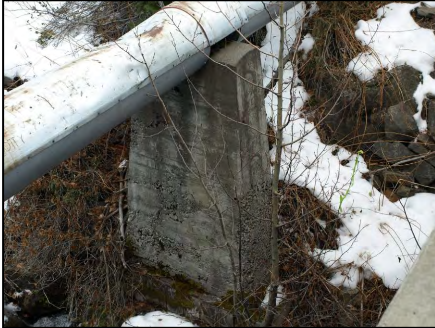
Figure 7.28. East side pier; photo taken from the Forest Service bridge. The case concrete pier tapers from its 6' x 4' foundation to a 36" x 15" top. Height from the top of the foundation to the top of the pier is 10' 6". The dent in the jacket is thought to have resulted from a falling tree.
