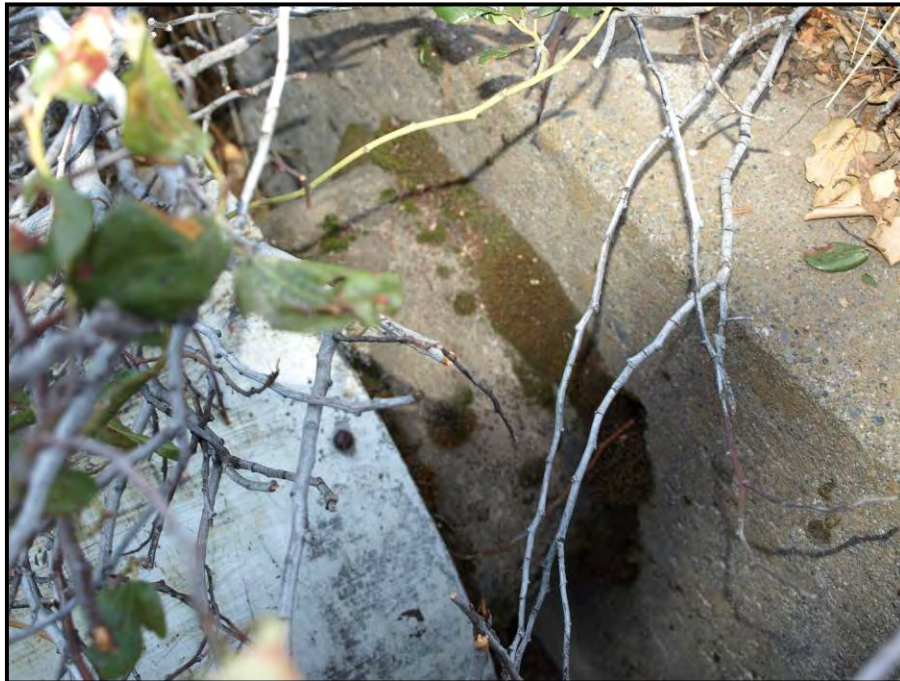
Figure 7.27. West side abutment showing 14" steel pipe leaving the portion fitted with the sheet metal jacket and insulation and entering the concrete abutment.
