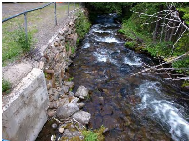
Figure 7.20. Retaining wall and fill on north side of creek below the dam, from 1967 plans.
