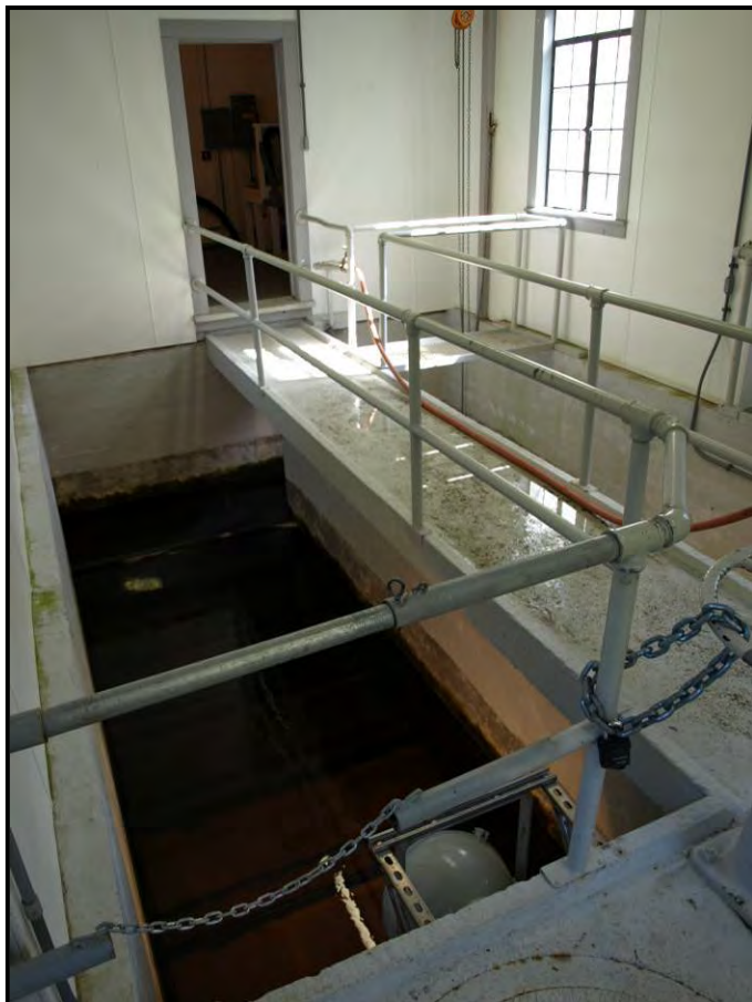
Figure 7.7. View of screen chambers, west chamber in foreground, looking north. The water enters at the bottom of the chambers at the south end, where the viewer is standing. It then wells up through the screens and leaves the chambers at the north end, where it enters the pipe to the reservoirs in Bend.
