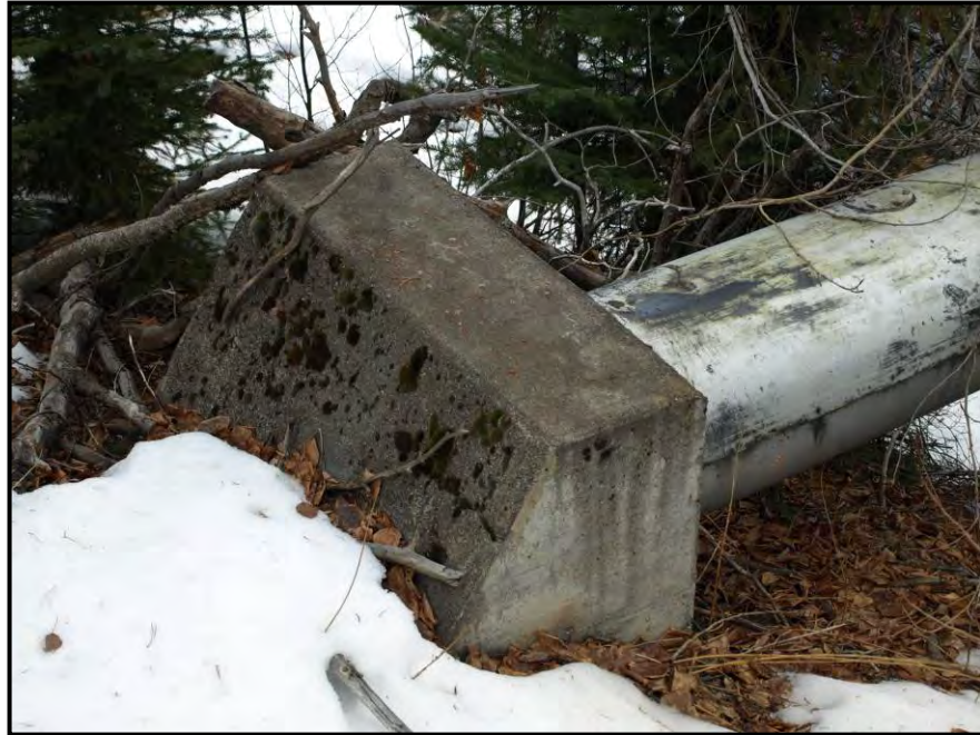
Figure 7.26. West side abutment showing pipe in sheet metal jacket emerging from the concrete abutment.
