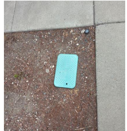
Irrigation valve box
