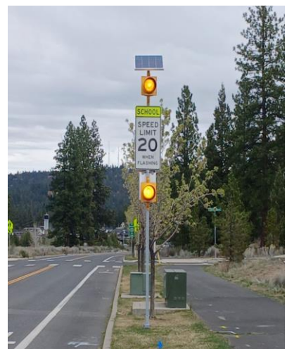
Signs, transformer, telecoms
