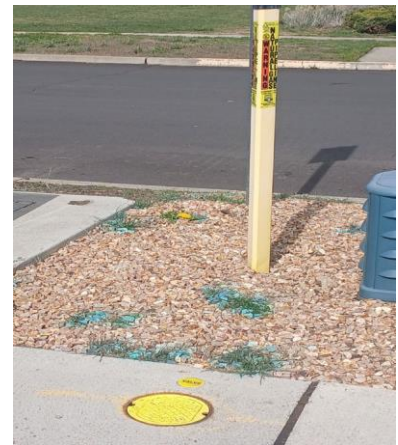
Gas valve & gas line marker
