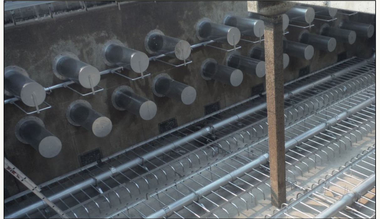
Pictured: Aeration Basin 3 IFAS Zone (1SCAP Project)
