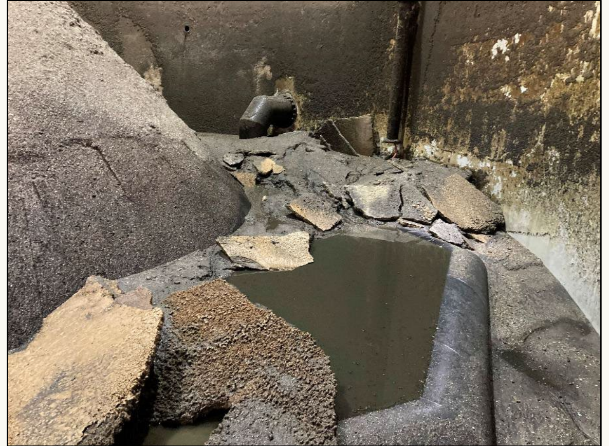
Pictured: Struvite interior wall slabs collapsed in Digester 3
