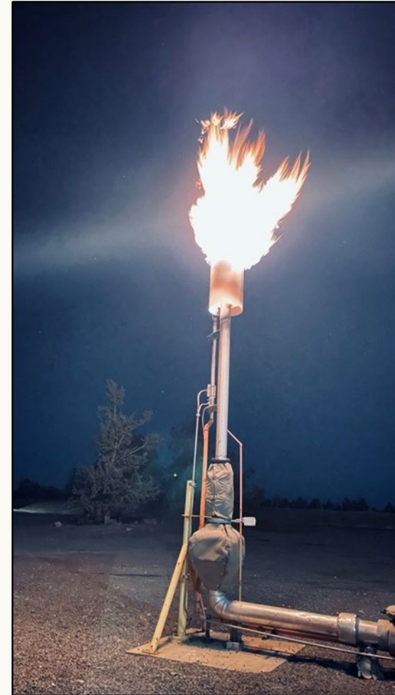
Pictured: Digester Gas Burner
